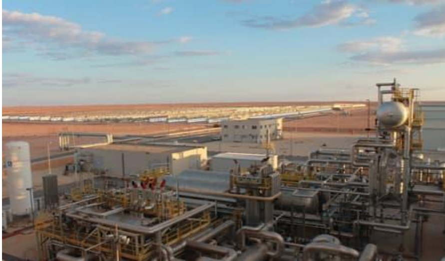
Figure I.4: Station de compression d'HASSI R'MEL.
